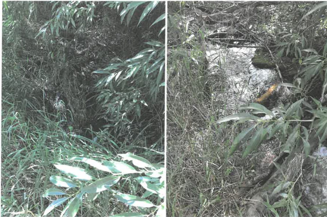
Photo Point 5 – Culvert under McDonald Road Photo Point 6 – Stream flow into pond
